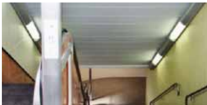
45° corner mounting for illumination of escalators and access passageways.
